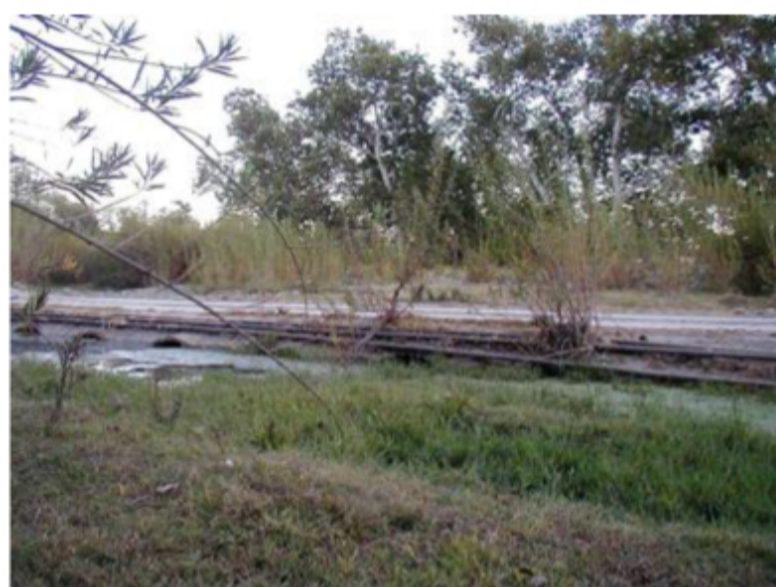
Photo #2. A level concrete ford is shown to the left and above. There are ten or so corrugated ~3-foot diameter pipes embedded in the concrete roadway. One can just barely see the tops of these pipes. The pipes are completely full of gravel.
